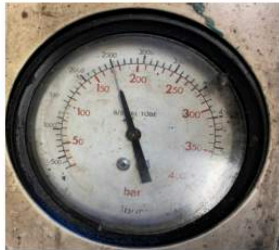
Fig 24: Pressure gauge shows 170 bar
